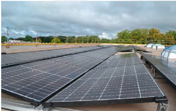
Detailed view of the solar modules with IBC AeroFix flat roof evaluation
